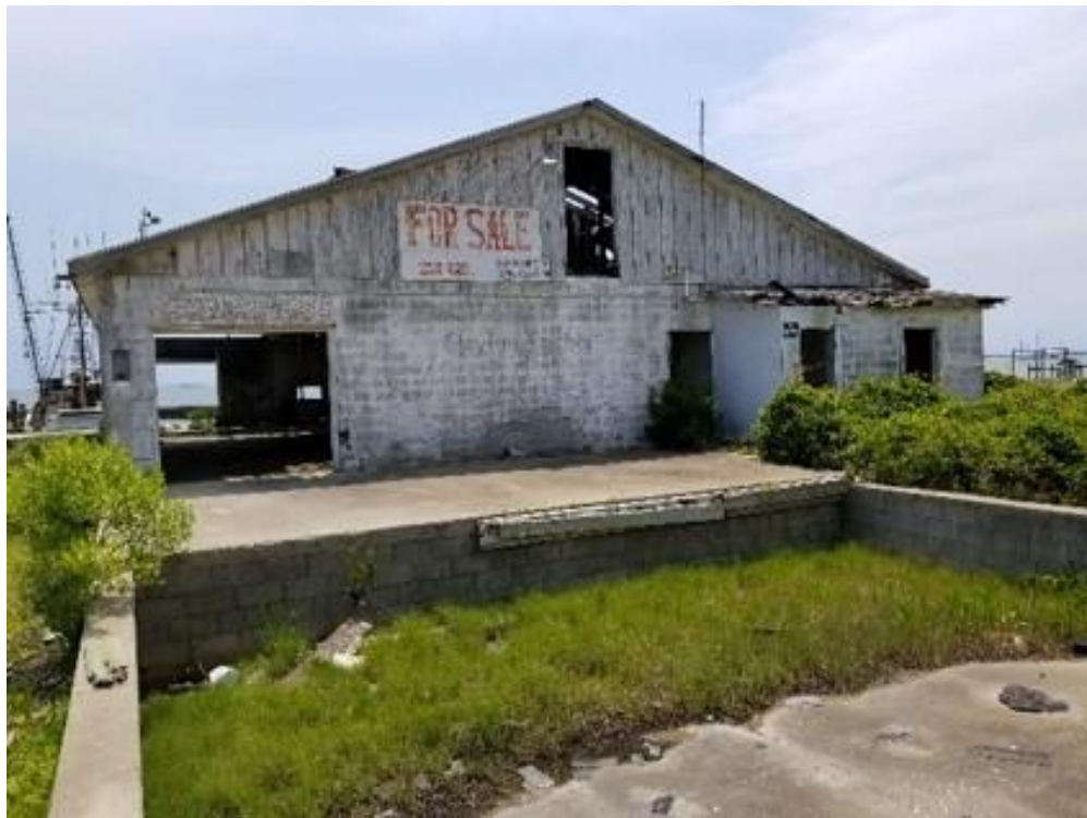
Figure 124. Front entrance of the dilapidated Old Fulcher fish house in Harker’s Island built in 1940s (Photo by Lynn Harris, ECU).
