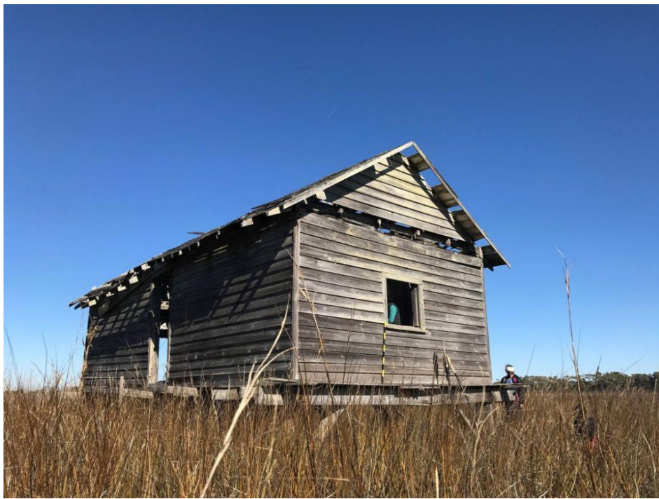
Figure 117. South and west face of boat house (Photo by Aleck Tan, ECU)
