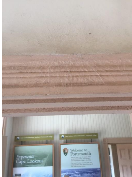
Figure 92. Ceiling example in the 1st floor entrance way of the Life Saving Station (Photo by Paul Willard Gates, ECU).
