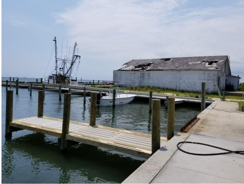
Figure 125. Roof damage of the dilapidated Old Fulcher fish house in Harker's Island built in 1940s (Photo by Lynn Harris, ECU).
