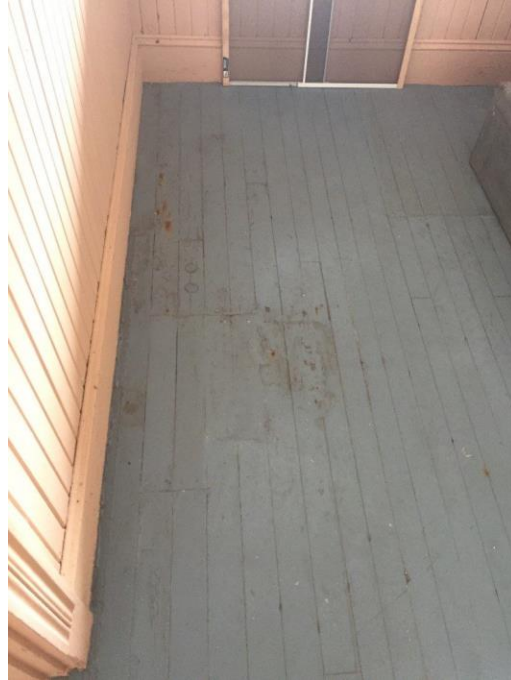
Figure 94. Floor example in the 1st floor pantry of the Life Saving Station. (Photo by Paul Willard Gates, ECU).
