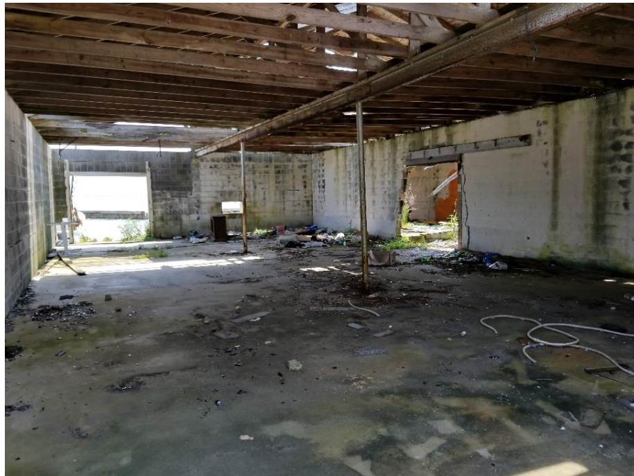
Figure 126. Interior damage of the dilapidated Old Fulcher fish house in Harker's Island built in 1940s (Photo by Lynn Harris, ECU).
