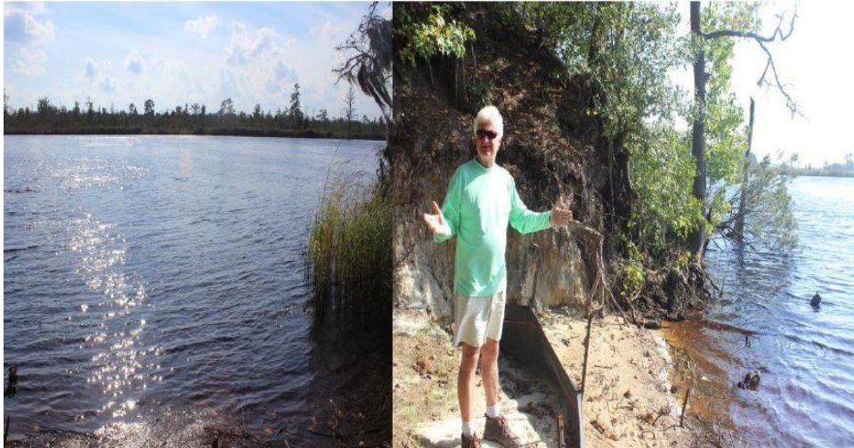
Figure 155. Boat Ramp in progress that may impact the shipwreck site with boat traffic and wake (Photo Lynn Harris)
