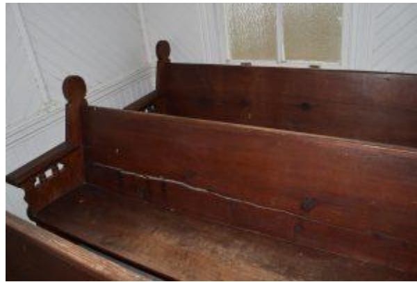
Figure 97. The current extent of damage to the backrest of a pew (Photography by Lynn Harris). Post Office and General Store
