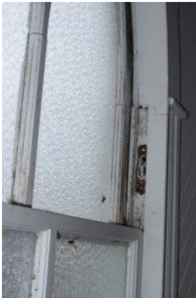
Figure 96. Example of window fixture corrosion, wasp infestation, and paint chipping on the interior (Photography by Lynn Harris).
