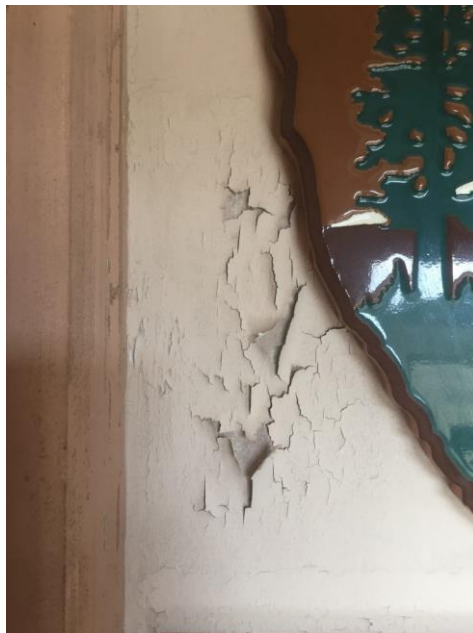
Figure 93. East wall example in the 1st floor entrance way of the Life Saving Station. (Photo by Paul Willard Gates, ECU).
