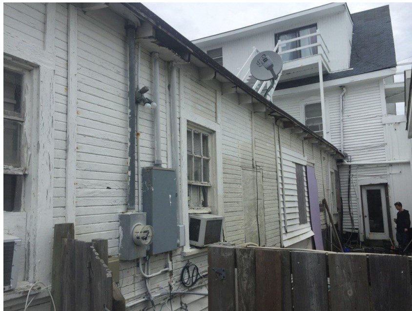
Figure 91. Rear: southern elevation of early twentieth century beach resort (Photo by Paul Willard Gates, ECU)
