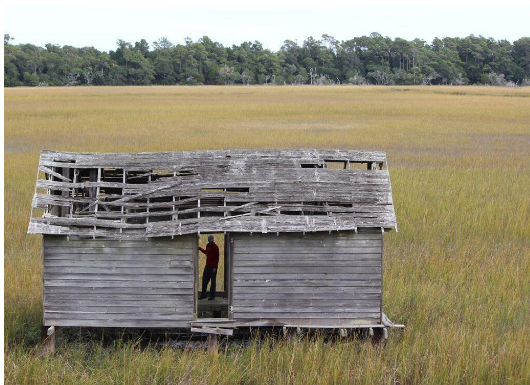
Figure 10. Aerial image showing deterioration of the roof structure of the boat house (Photo by Lynn Harris)
